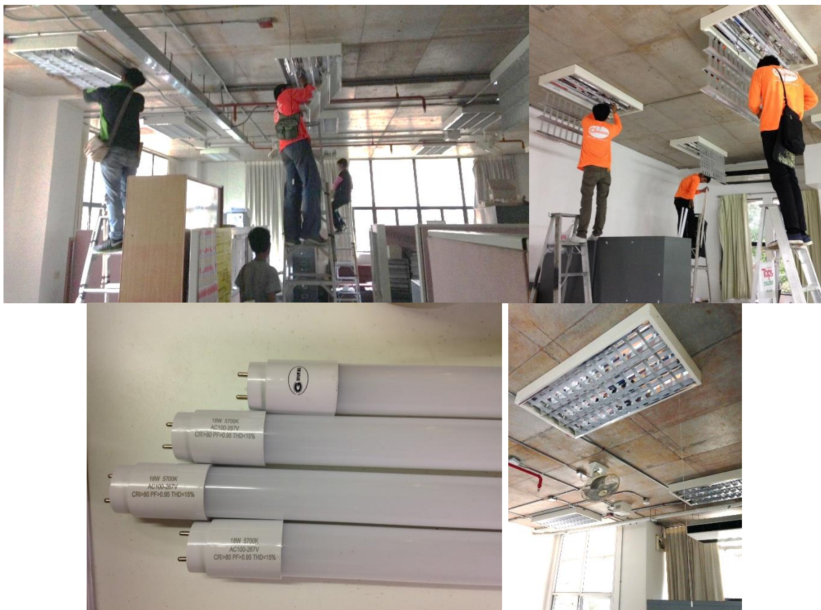
รูปที่ 2. 26 LED lighting fixtures are replacing conventional appliances (individual adjustment in all fixture)
