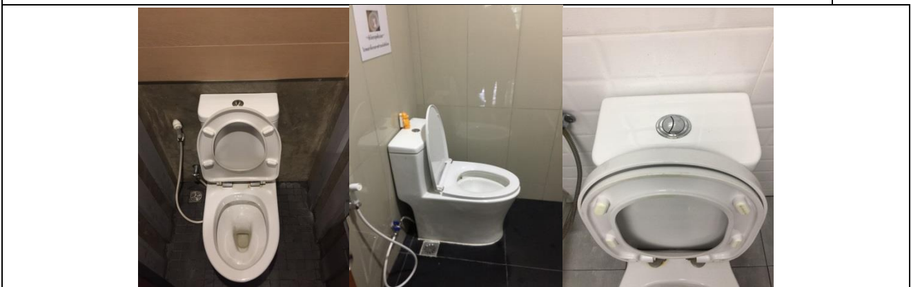
A water efficient water closet (toilet) at the Faculty of Architecture Building (left) at Faculty of Sciences Building (center) and at Art Gallery (right) [Project-1]
