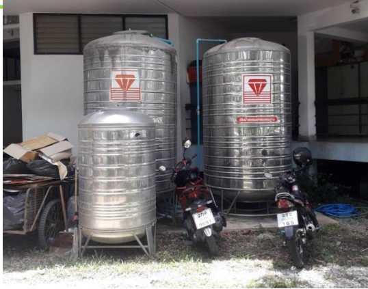
Examples of two 2,500- litre rainwater tanks at the Administration Building, the CMU Demonstration School
