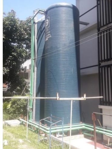
Examples of a 5,000-litre rainwater tank at the 55-year Nursing Building
