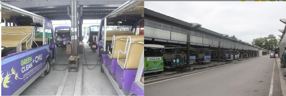
Electric shuttle trolleys charger stations
