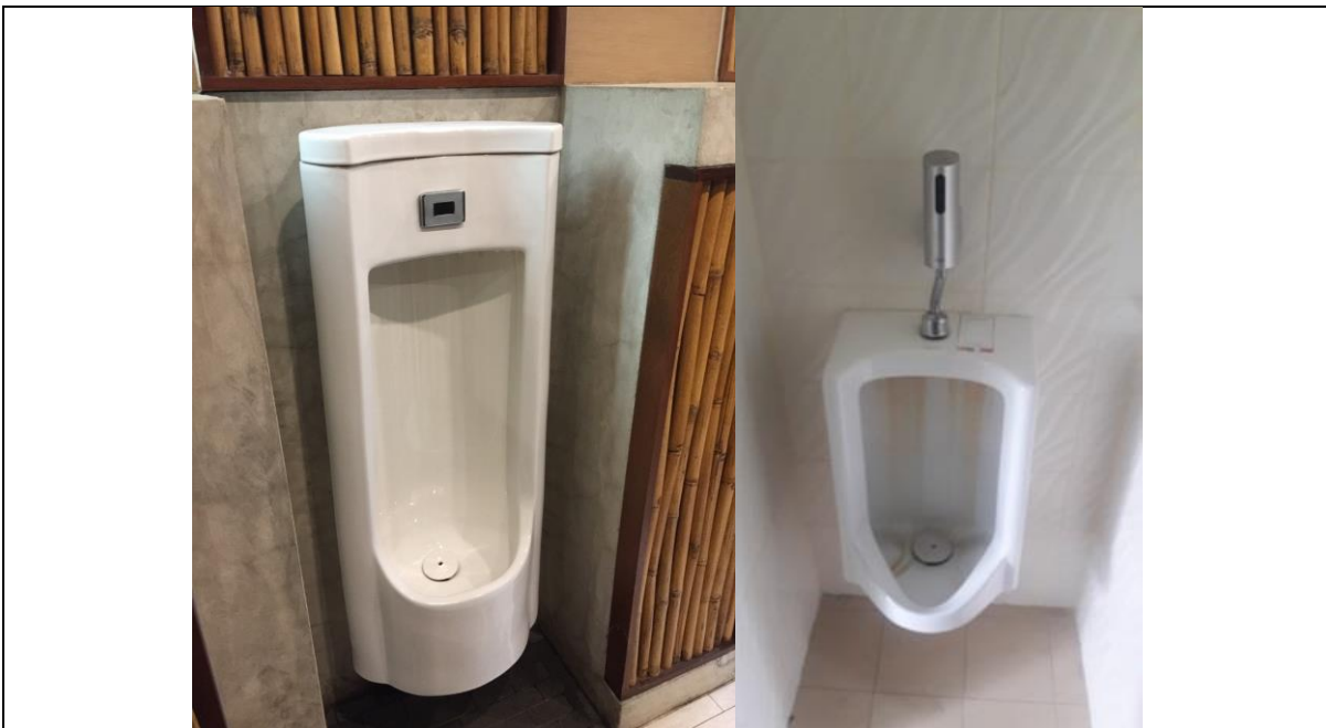
Automatic urinal at the Faculty of Architecture building (left) and at the Department of Community Medicine Building [PROJECT-1] (right)
