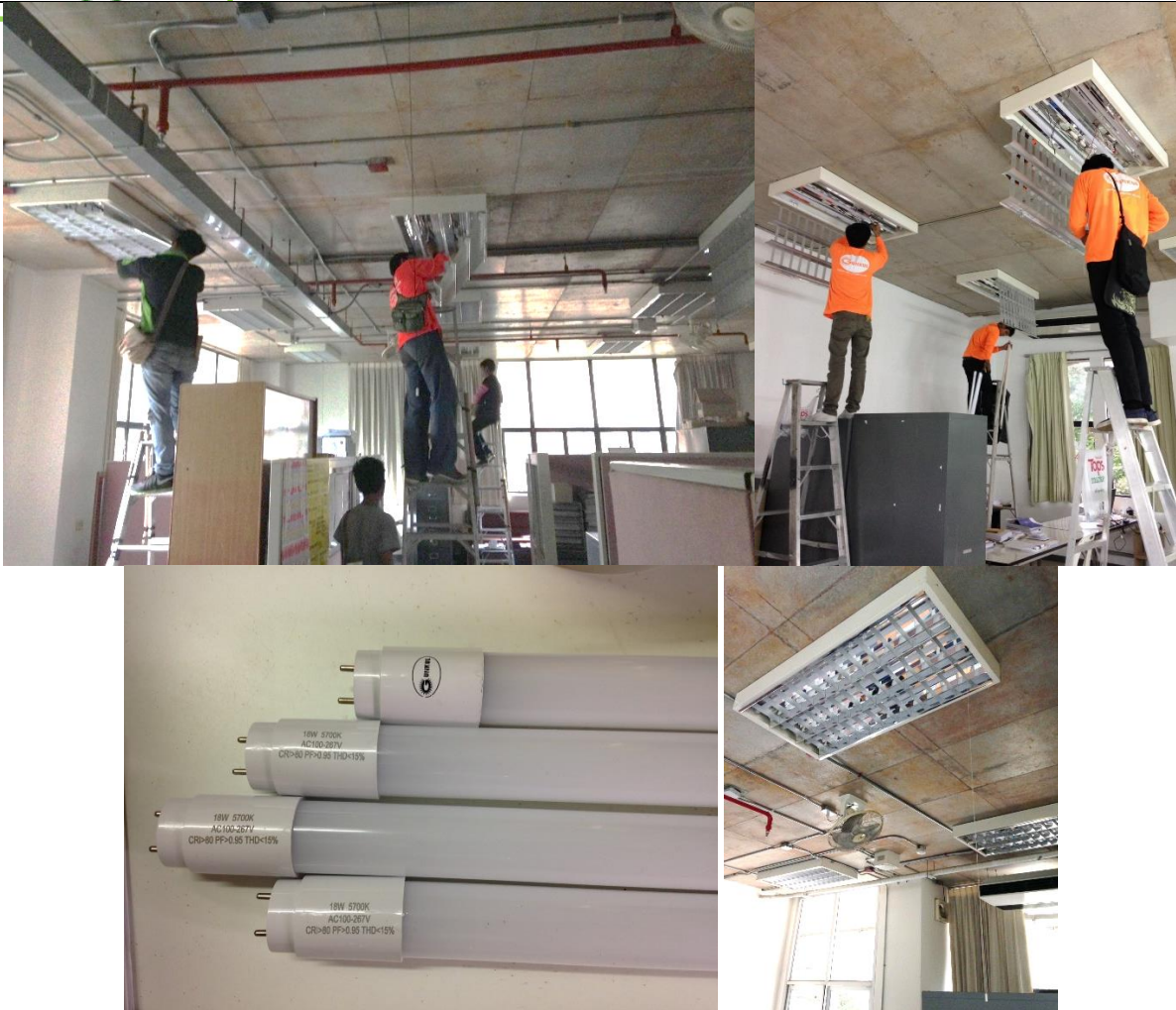
LED lighting fixtures are replacing conventional appliances (individual adjustment in all fixtures)
