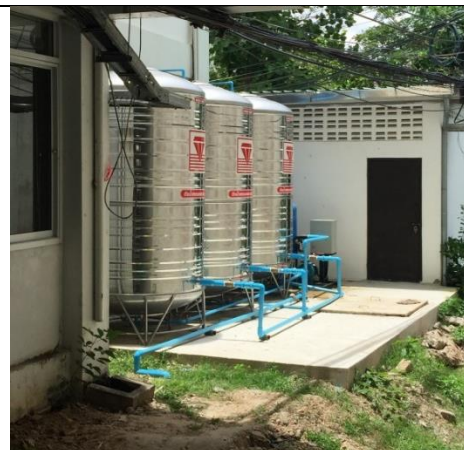
Examples of three 4,000-litre rainwater tanks at Learning center Building RB5
