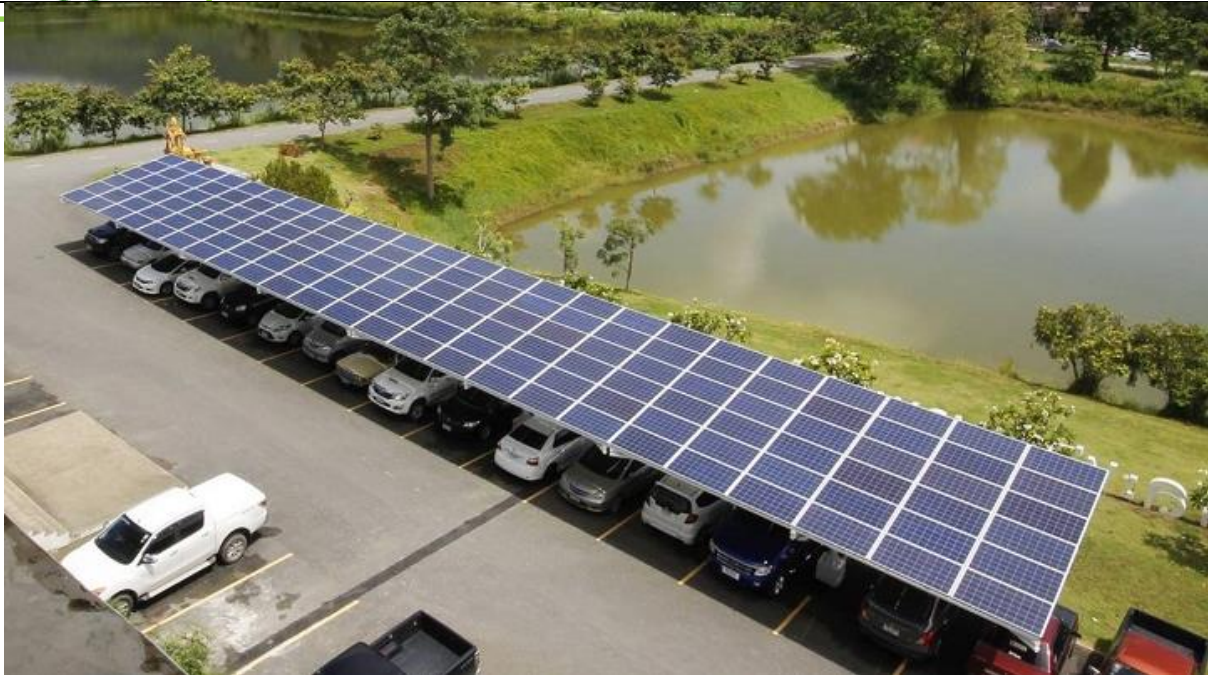
Solar Parking Canopies, CMU (Source: CMU, taken on 15 Feb 2018)
