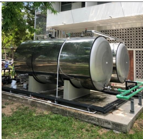
Examples of two 5,000-litre rainwater tanks at Male Dormitory 5
